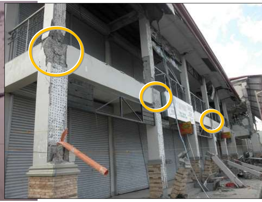
A market building affected by Bohol EQ 2013 in the Philippines
