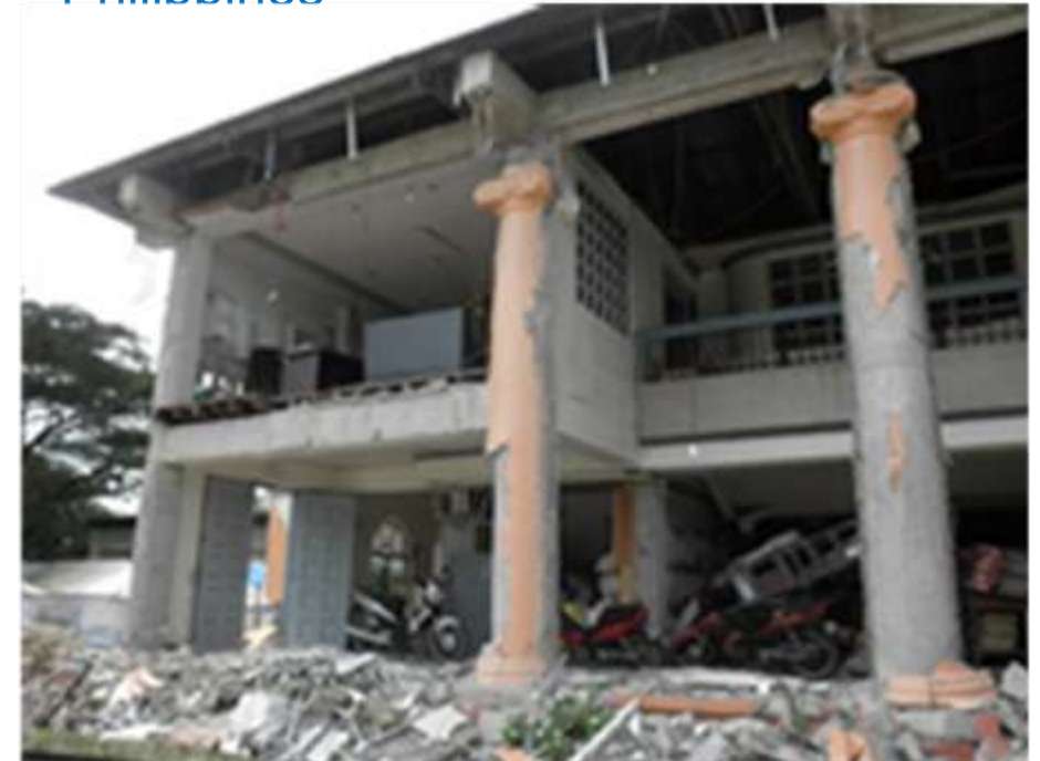
A municipal government building lost most of cladding walls by Bohol EQ 2013, in the Philippines
