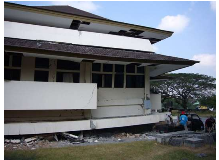
Failures in columns on the ground floor
