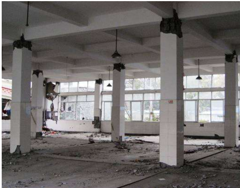
A school building affected by Wenchuan EQ 2008 in China
