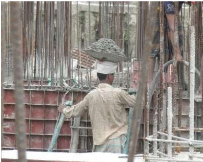
A poor practice in developing countries: workers just throw concrete into form panels
